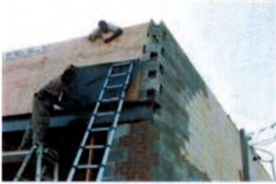
Charles Holland, left, and Sam Jones work on the building facade that is slated to become the location for Brown Bag Productions in the historic Burlington neighborhood of East Knoxville on July 13, 2016. (AMY SMOTHERMAN BURGESS/NEWS SENTINEL)
